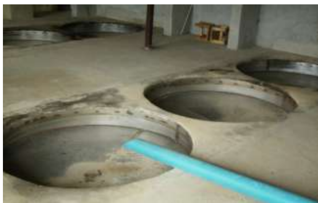
Fig. 6: Underground Firing Evaporation System
