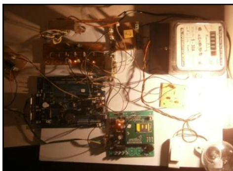
Fig 4: GSM based pre-paid remote energy meter when the power is ON
