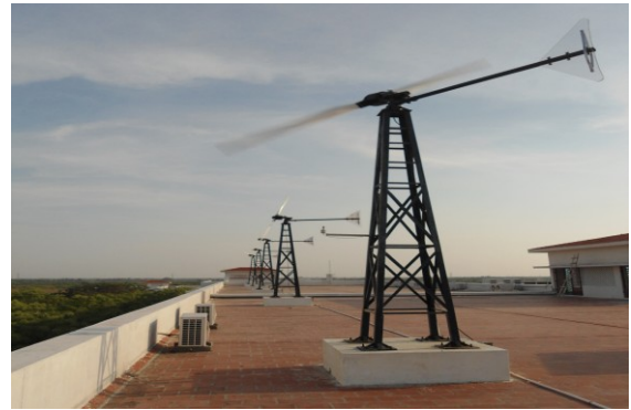
Fig 2.view of wind section
