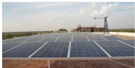
Fig 3.view of solar section
