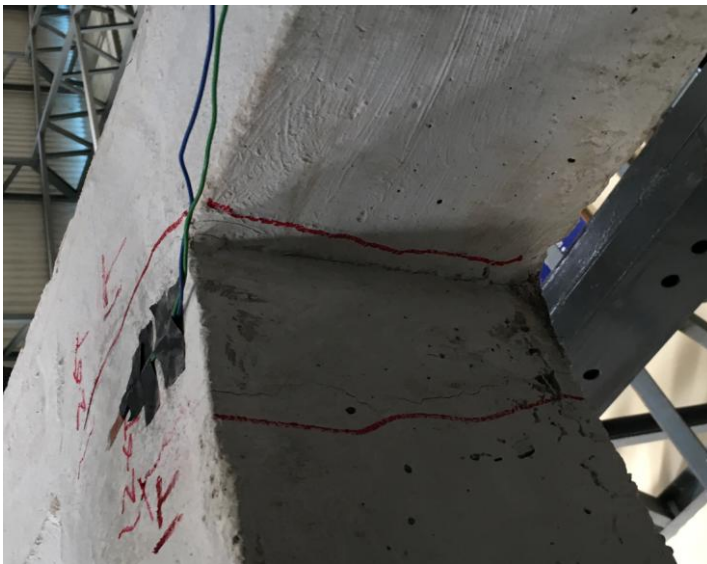
Figure8: Crack pattern of SFRC Beam column joint
