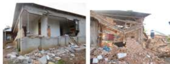
Fig. 1: Buildings damages in Bukoba following magnitude 5.9 September 2016 earthquake
