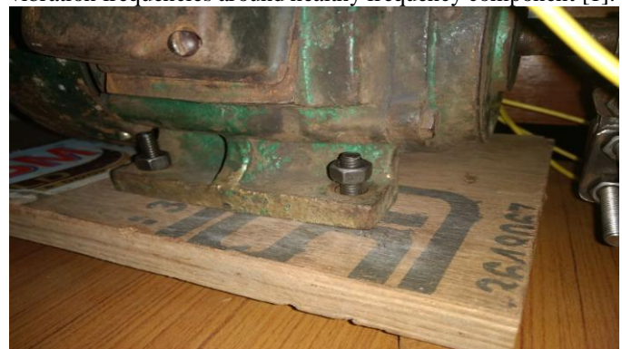
Fig.4: Loose mounting condition.
